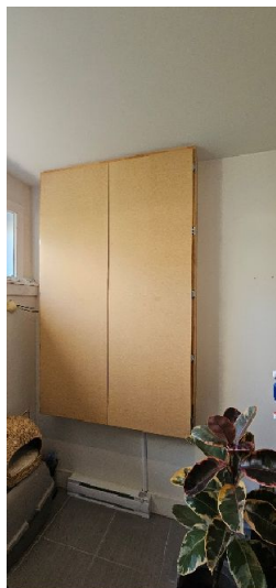
Distribution panel (1) No major anomalies Basement
