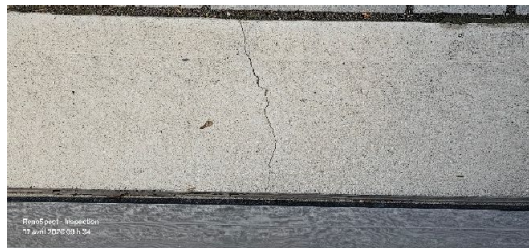
Masonry lintel Damage observed (2) Garage door
