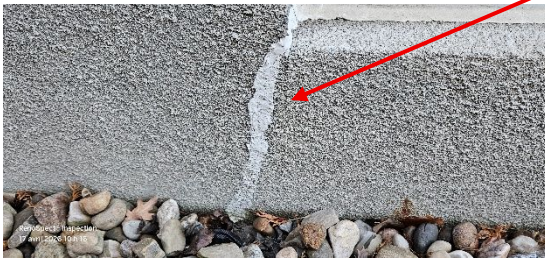
Foundations Observed crack (-3mm / 1/8 inch) Window (bottom) - Left side
