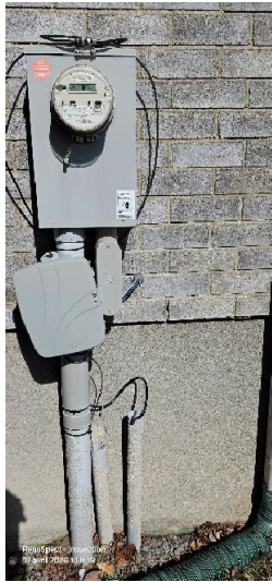
Main electrical entrance - Underground Left side (front)
