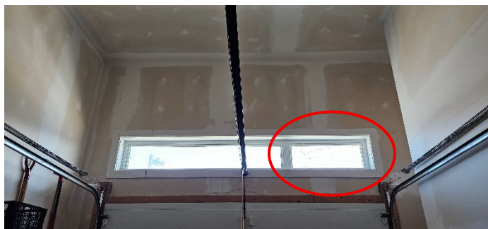
Interior windows Broken thermos glass Garage
