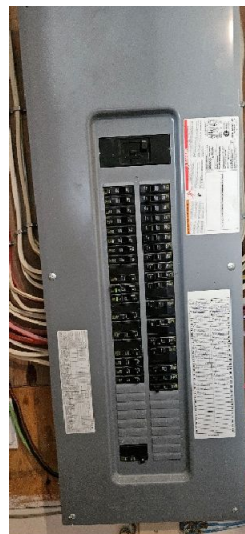
Distribution panel (2) No major anomalies Basement
