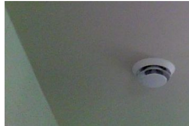
HRV – Ceiling Fan No major anomalies Bathroom
