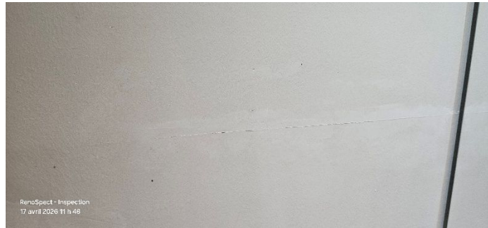
Wall finishing coating Repair observed Bathroom
