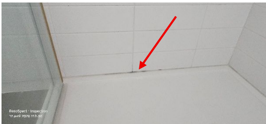
Appliances and taps Sealant missing or damaged Shower
