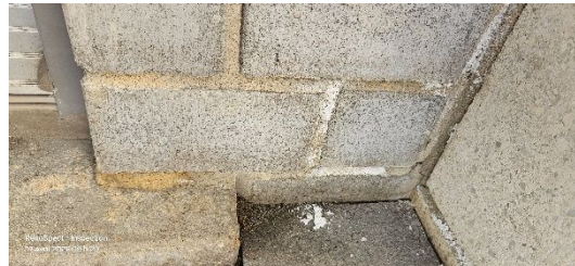
Entrance balcony - Efflorescence observed Front facade
