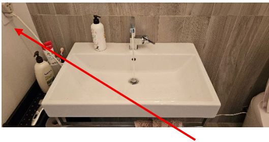
GFCI outlet malfunction Bathroom
