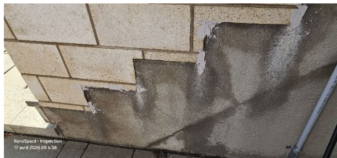
Entrance balcony - Infiltration Front staircase
