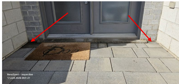
Entrance balcony - Water accumulation/infiltration Front facade
