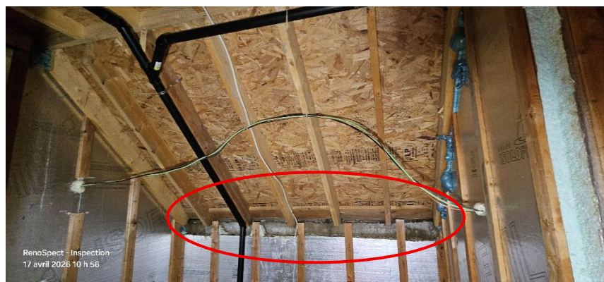
Cold room – Signs of leakage Basement (front)
