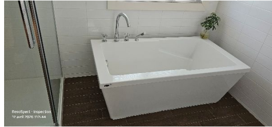
Appliances and taps Sealant missing or damaged Bathtub
