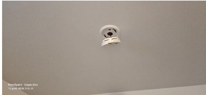
Fire alarms Absent or non-compliant
