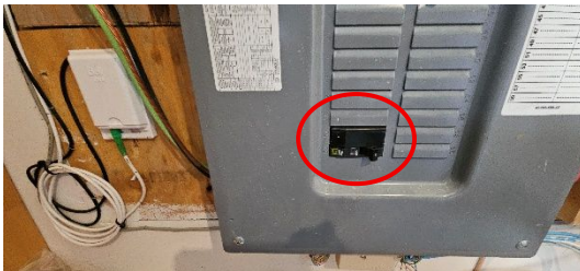
Charging station Without any anomalies 60A / 240 Volt Circuit Breaker
