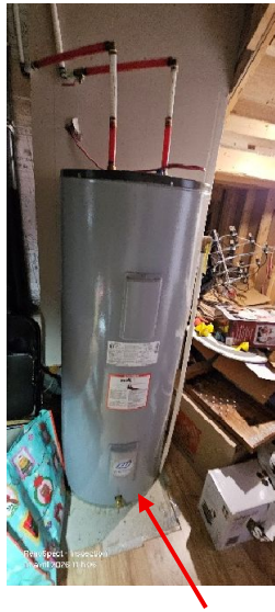
Water heating system Inadequate connection to the floor drain (Mechanical chamber)
