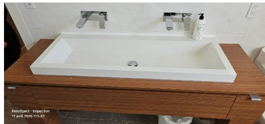
Appliances and taps Sealant missing or damaged Sink
