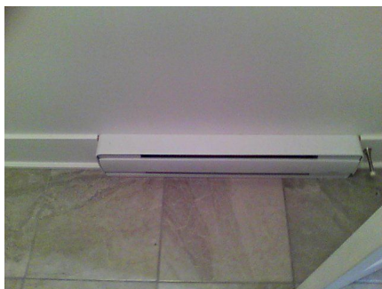
Heating appliances - Electric baseboard heaters ( Num ) Basement
