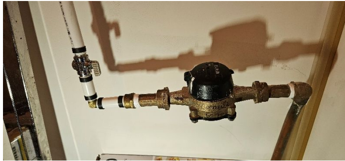
Main entrance Water meter Basement
