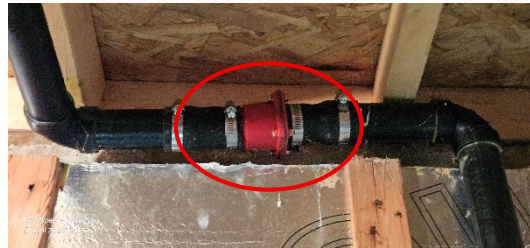
Check valve No major anomalies Cold room
