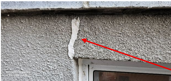
Foundations Observed crack (-3mm / 1/8 inch) Window (top) - Left side
