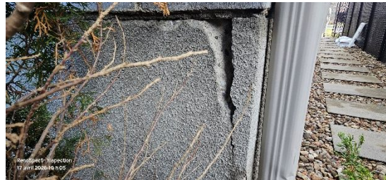
Foundations Crack Observed (+3mm / 1/8 inch) Back left corner
