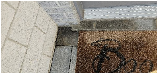
Entrance balcony - Damp patch Front facade
