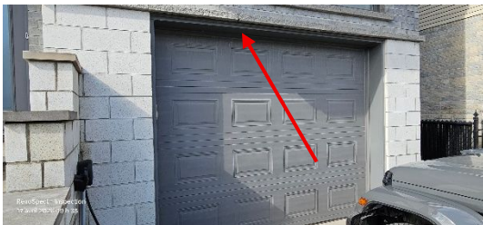
Masonry lintel Damage observed (1) Garage door
