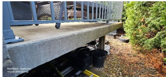
Earthworks and landscaping Incomplete installation Backyard
