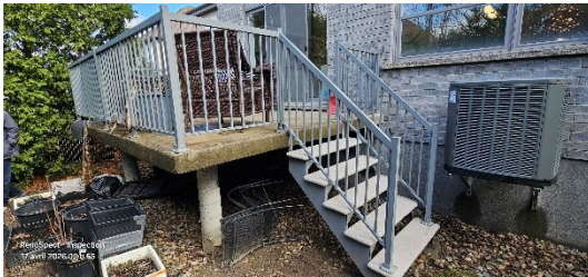
Exterior stairs (1) Inadequate anchoring Rear balcony
