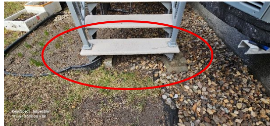
Exterior stairs (2) Inadequate anchoring Rear balcony
