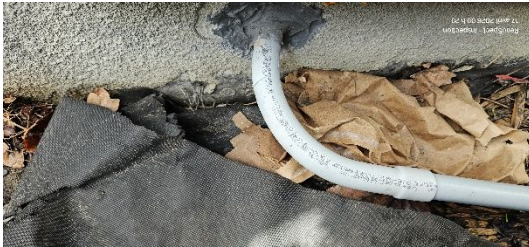
Charging station Without any anomalies Supply conduit
