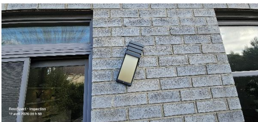
Light fixture - Inadequate mounting Rear facade
