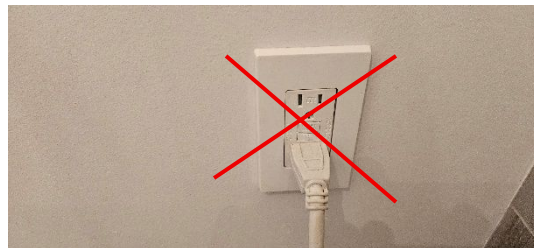
Plug into a GFCI outlet - DANGER Bathroom
