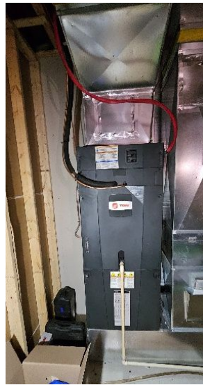
Central heating appliances Basement
