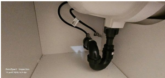
Drainage pipes (ABS) No major anomalies Sink
