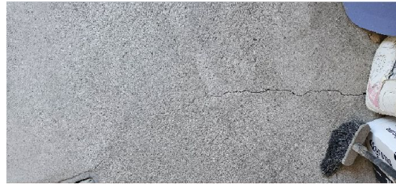
Concrete slab Cracks observed Garage
