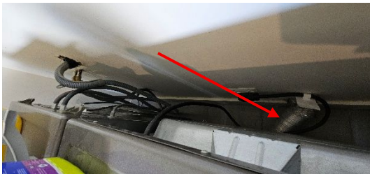
Dryer vent - Aluminum No major anomalies Basement
